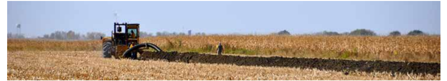
▲ Installation of a controlled drainage system on a family farm. © NRCS/SWCS photo by Lynn Betts
