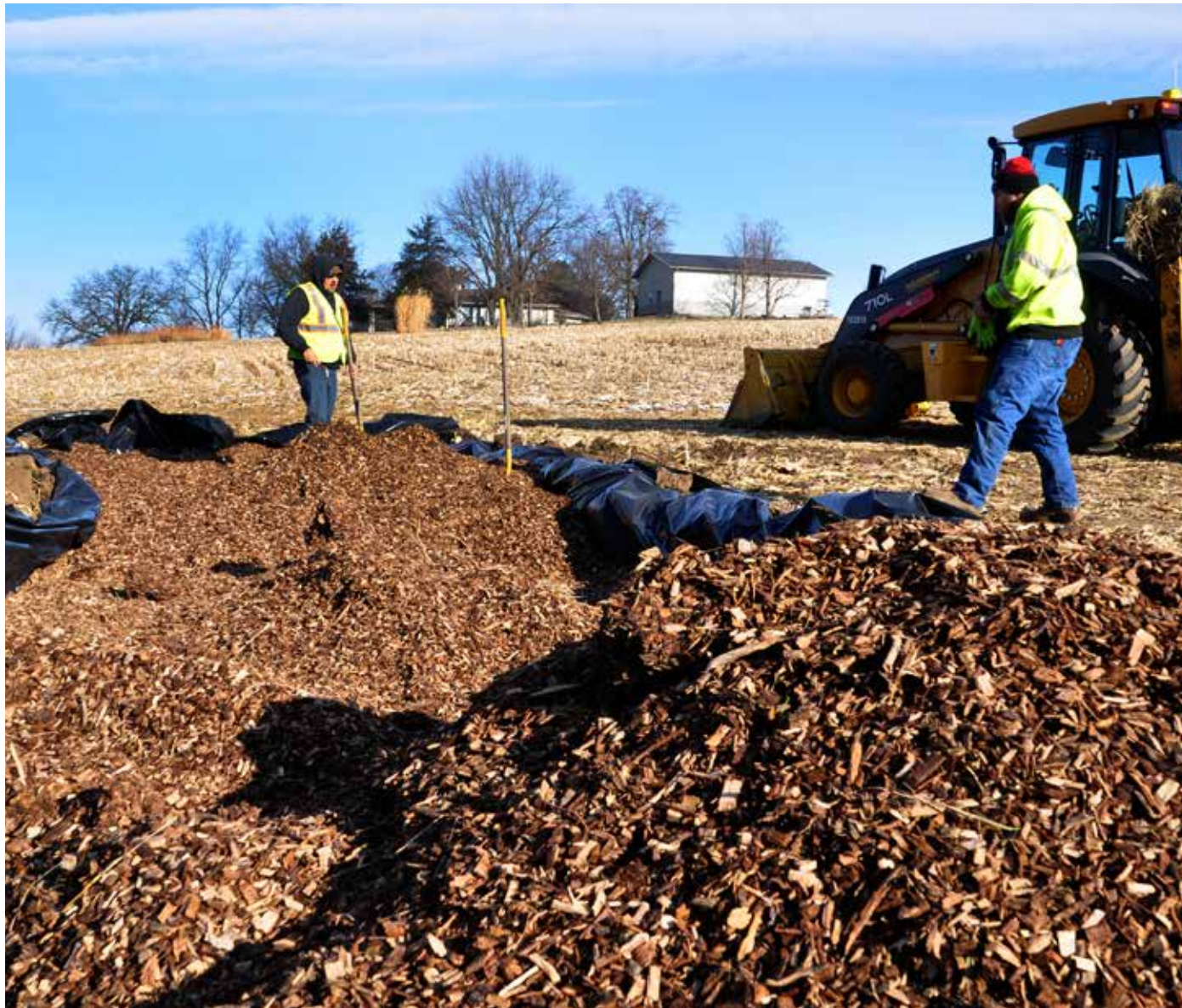
▲ The installation of a wood chip bioreactor. Wood chips remove nitrates from tile water as the water flows through the bioreactor. © SWCS/IDALS Photo by Lynn Betts
